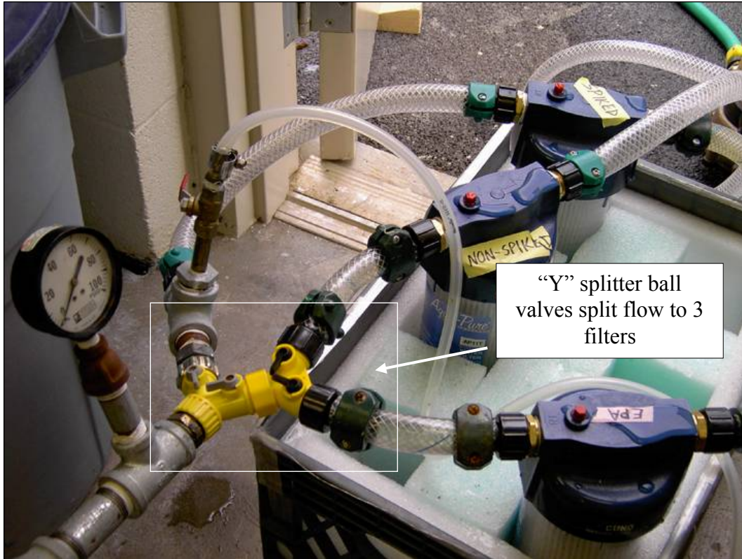
Figure 4-3. “Y” splitter ball valves were used downstream of the pressure regulator to split the flow to each filter.
